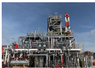
Pilot facility to produce ethylene from renewable ethanol
