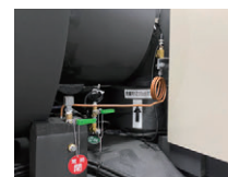
HFO (R1233zd) refrigeration equipment
