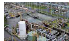
Activated sludge treatment facility
